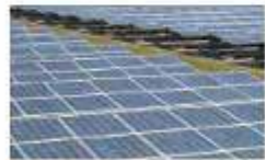
roof mounted PV arrays
